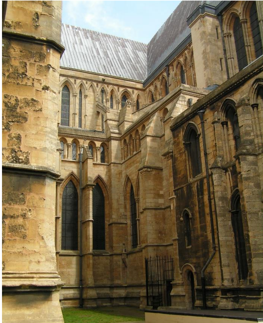
Figure 3: Lincoln Cathedral between the Women's Chapel and the Song School. Stonework in the foreground shows biological patina (dark stains) and damage, stonework in the background has been recently cleaned. On the left hand wall biological growth and spalling of the stone work are evident, especially where overhanging stonework provides a protective environment; this is especially clear at the bottom of the wall where there is a clear gradient between patinated stone and clean stone moving down from the overhang. On the right hand of the image, the Song School, water flow down the wall due to insufficient guttering, and shelter of the courtyard, has led to a damper environment than that on the left, patina is clearly evident working from the left near the door across towards the gutter downpipe where a combination of improved guttering and lead salts, which can be seen as a slight greying of the stone behind the downpipe itself, have led to a reduction in biological growth.
