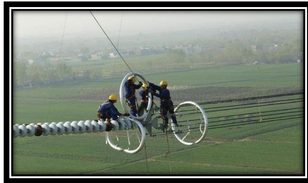
Figure 91 Workers upgrading ultra-high voltage lines on April 13, 2011 in Henan Province's Nanyang region. Source: http://en.people.cn/102774/7680026.html
