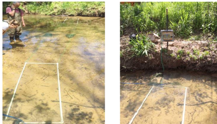
Figure 2.5: Photos showing the half duplex antenna systems installed in Raccoon Creek to monitor fish movement.
