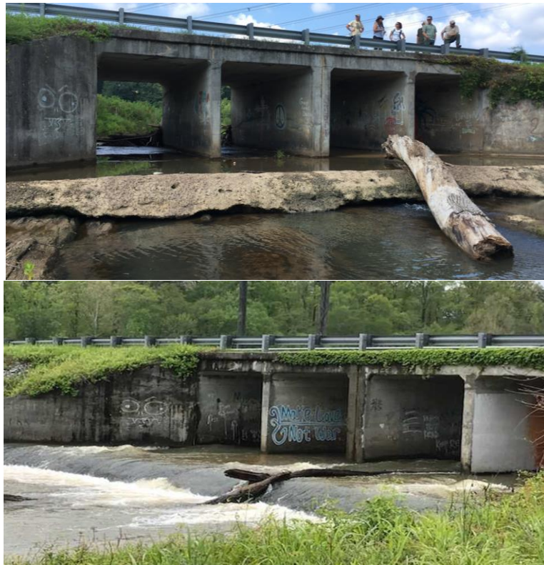
Figure 2.1: The culvert at Raccoon Creek Road during low flow (top) compared to high flow (bottom).
