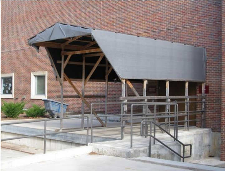
Loading dock canopy built for SCRC move. Photo courtesy of Julie Mosbo.
