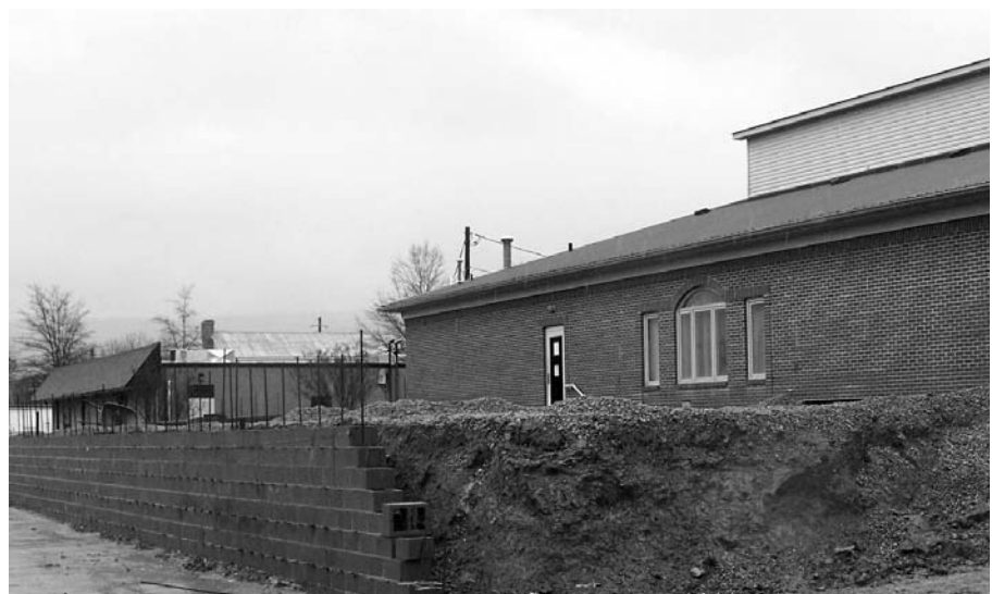
Construction and site work began just a few weeks ago at the Dade County Public Library in Trenton, Ga. This photo was taken five weeks into the project on Nov. 30. (Photo by Jeremy Hobbs)
