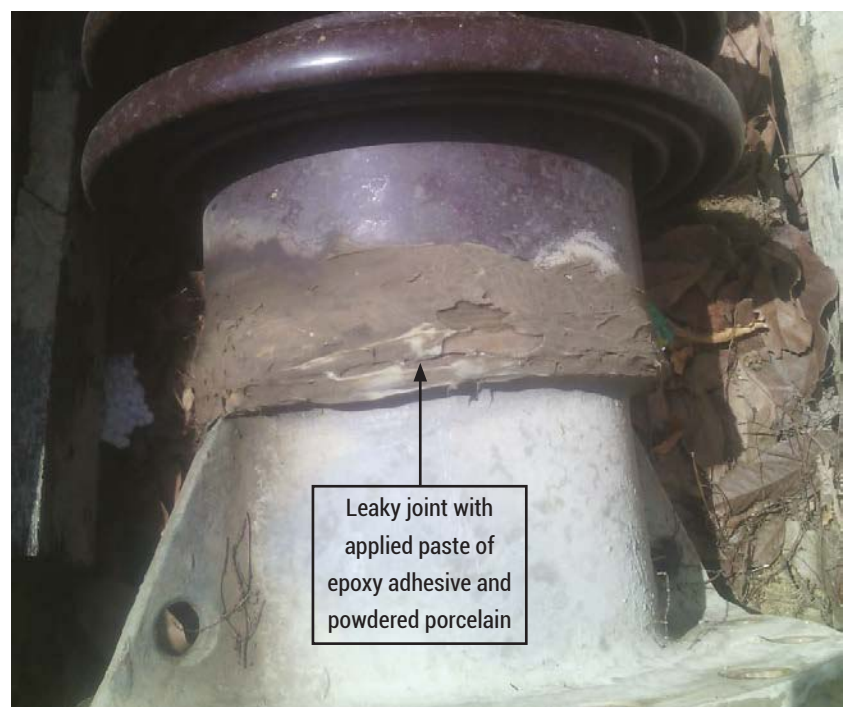
Figure 2. Leaky 245 kV OIP bushing of 1U- phase of the transformer with application of homogeneous paste of Araldite (epoxy adhesive) and the powdered porcelain.
