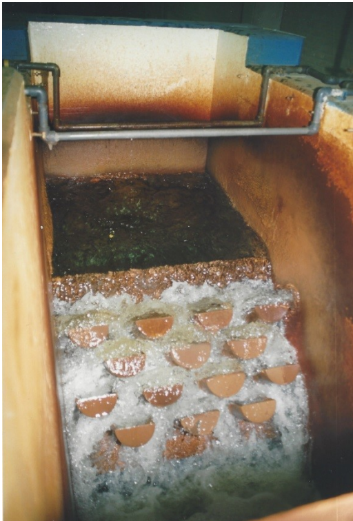
Fig. 6 Dosing of ferric chloride in a cascade
