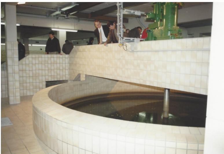
Fig. 7 Top: tapered flocculation tanks; Center: mixing device in flocculation tank; Bottom: flocculation tank in Wuppertal (Germany)
