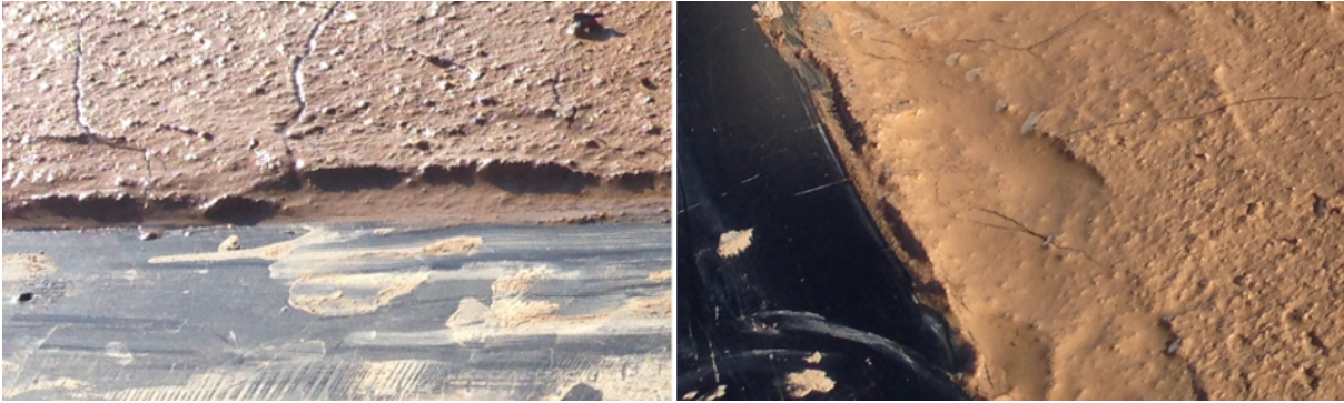
Figure 5.49. Thin cracks formed close to the lateral walls of the container at the start of the test.
