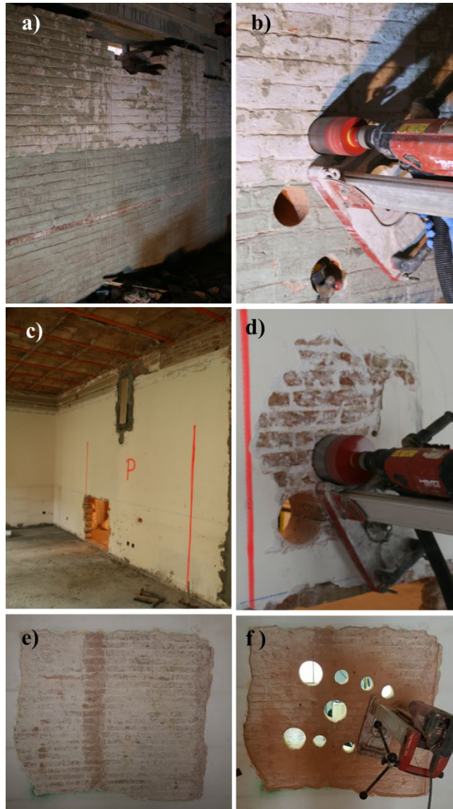
Fig. 8. a) Façade wall investigated in “Fabra i Coats” factory and b) in-situ core drilling for campaign “MB”, c) inner wall of the analysed building in Rambla Catalunya street and d) in-situ core drilling for campaign “MC”, e) inner wall of the building in Ciutat Vella and f) in-situ core drilling for campaign “MD”.
