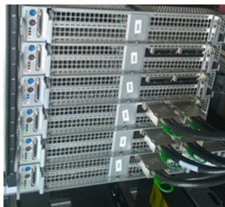
(b) Rack of servers with the corresponding PCI connections for the motherboards, each server is a GN node
