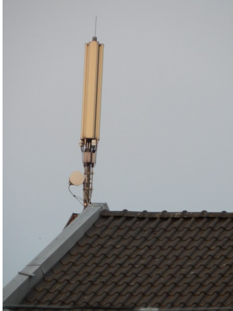
Picture 1.3. – An antenna for mobile communication on a roof. Photograph by author.
