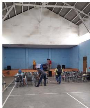
Figure 4. Community meeting place that needs renovation and structure strength investigation due to earthquake and landslide disaster occurrence
