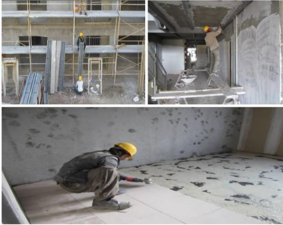
Fig. 1: Some jobs of construction industry involved in ergonomic risk factor assessment process.
