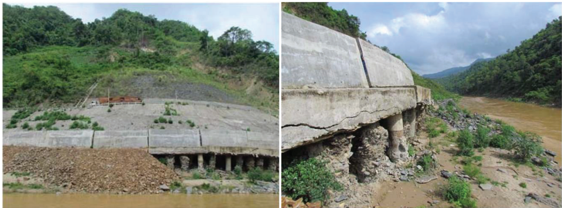
Fig.4. 28 The field photos of Loc.4 landslide: (Left) The boundary of the landslide with the surrounding rocks is quite clear. On the surface of the landslide body has been reinforced by stone masonry, but the sliding block shifted causing the surface to break. (Right) The concrete retaining wall at the foot of the sliding block breaks and moves toward the river.
