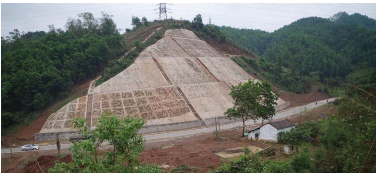
Fig.4. 79 Overview of the Km95 Landslide located at NH6 (photo taken in March 2014)
