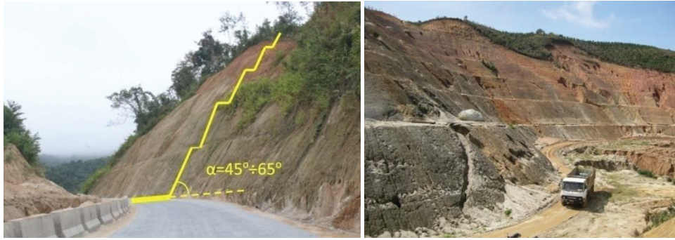
Fig.2. 28 Cross section of cutting road on HCMR (left) and East Truong Son route (right)
