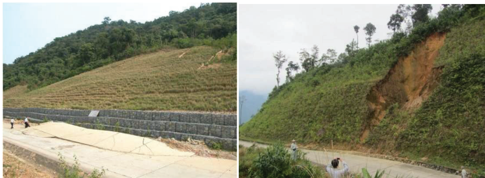
Fig. 3. 4 Landslides caused emerge of pavement (left) and Collapses (right) on HCMR
