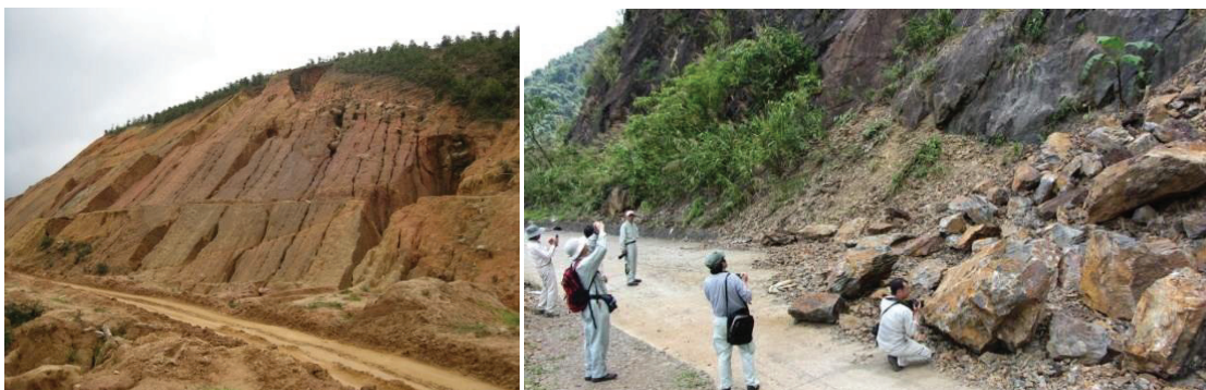
Fig. 3. 5 Erosion often occurred on Truong Son Dong route (left), Topples and rock falls on HCMR (right)
