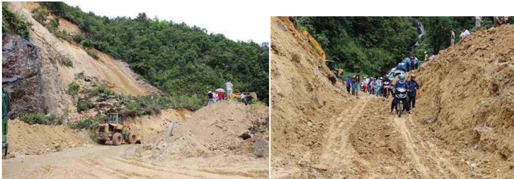
Fig.2. 7 Landslide on National Highway 4D (September 20 th , 2014)
