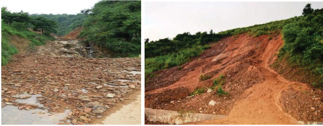
Fig. 3. 7 Flow landslide on NH34 (left) and on NH7 (right)
