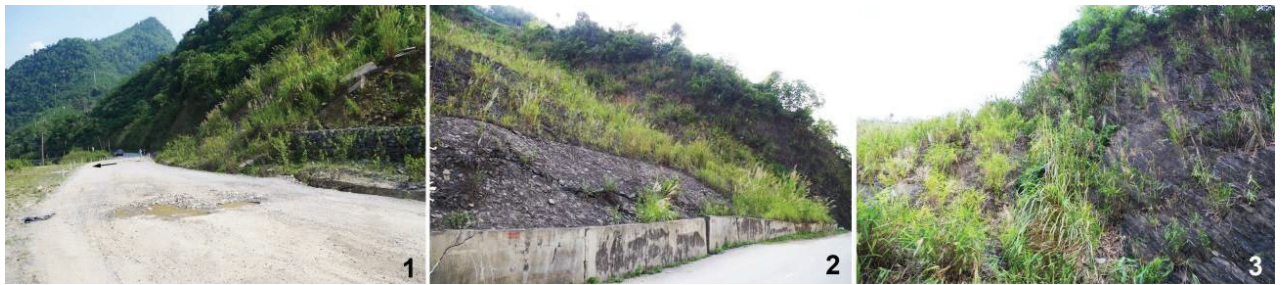
Fig.4. 13 Field photos at LS 2 in Fig. 4.: 1, The toe part of the landslide body deforms the road. 2, The body is pushing the retaining wall 3, The side boundary between the landslide body and non landslide slope.
