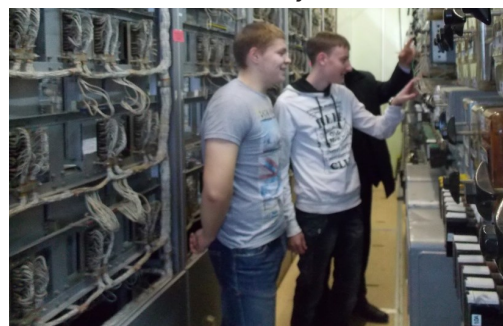
Pic. 3. Introduction to relay equipment.
