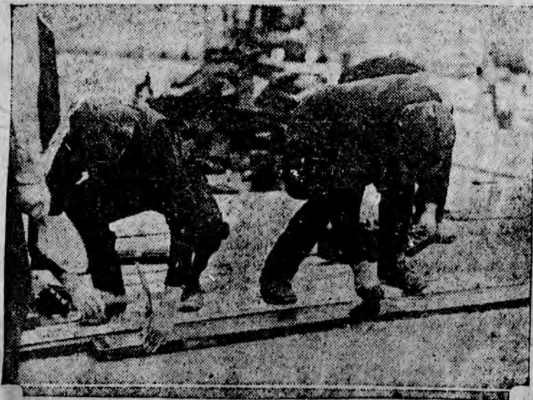
Workmen laying the new pavement in regular lines. The blocks are put in rows with the ribbed side downward and set in mortar. Beneath the thin layer of mortar there is a concrete base. In color the rubber blocks are of a dull black.
