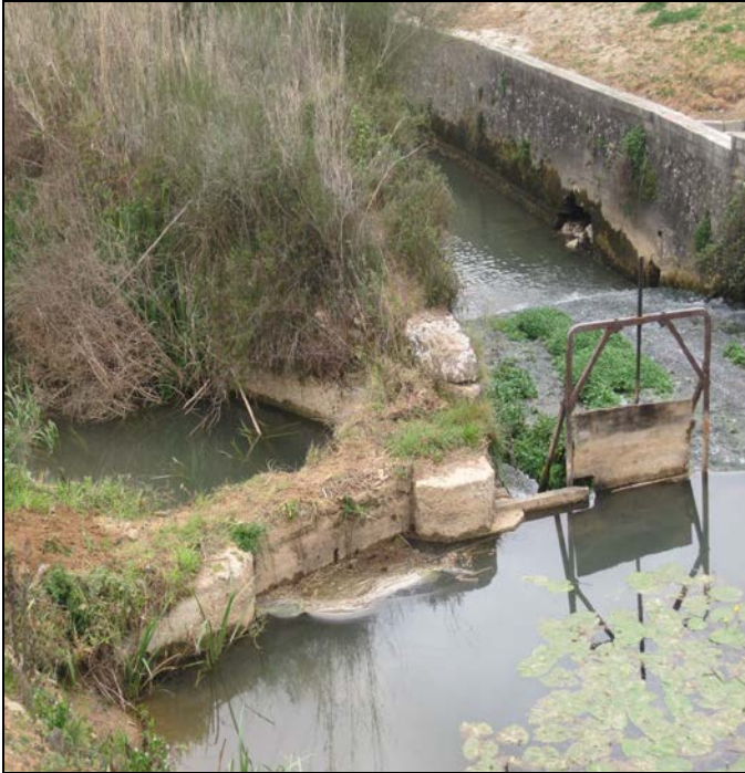
Fig. 2. Weir on the Alcoa river allowing the Abbey non-drinking water supply (V. F. Jorge).
