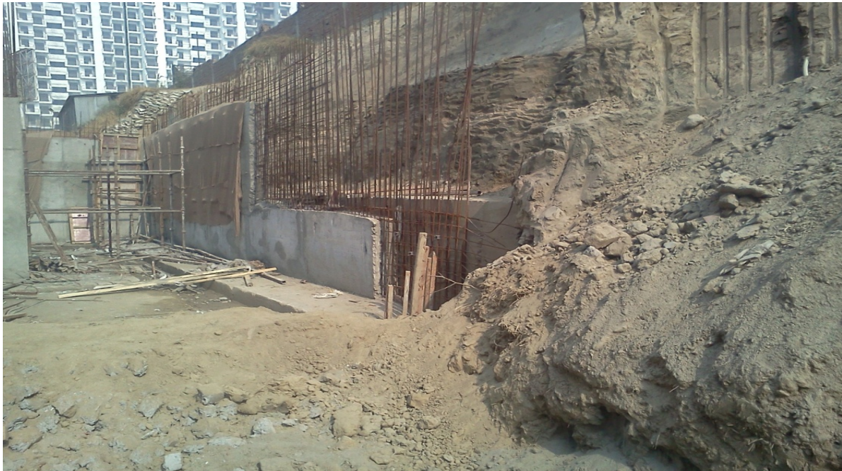
Figure 15. Collapse of soil during construction of retaining wall
