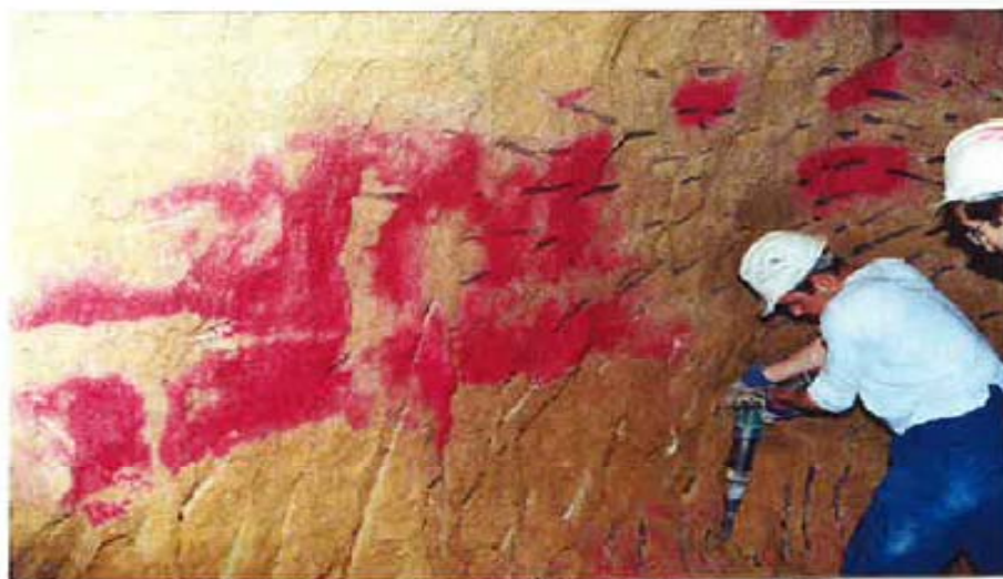
Figure 10. Ease of excavation due to grouting (pink in color) carried out prior to excavation
