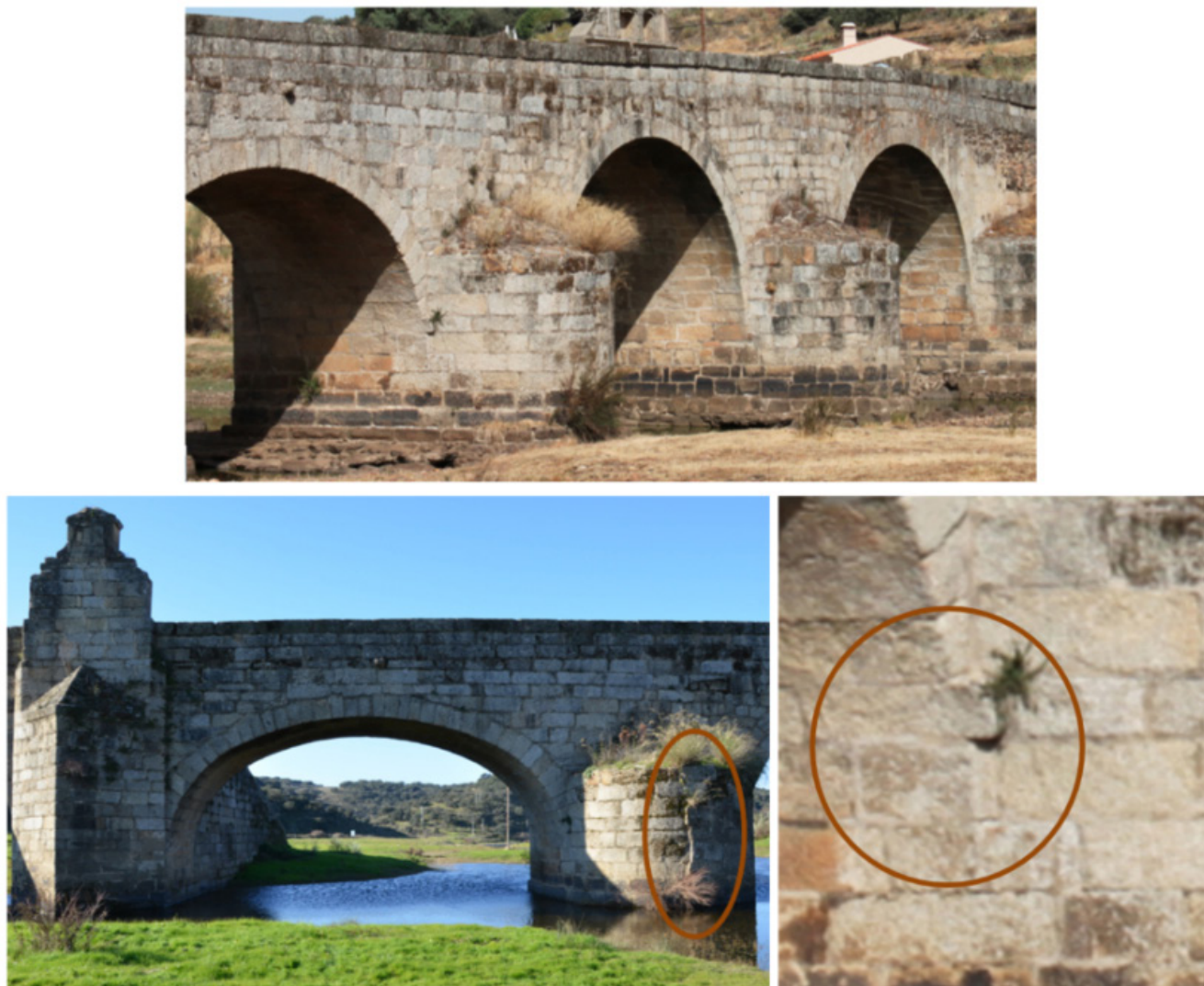
Figure 2. (Up) North Half of the Bridge, (down left) view of third arch and second breakwater with a break line, and (down right) detail of the Springer of the Third Arch.
