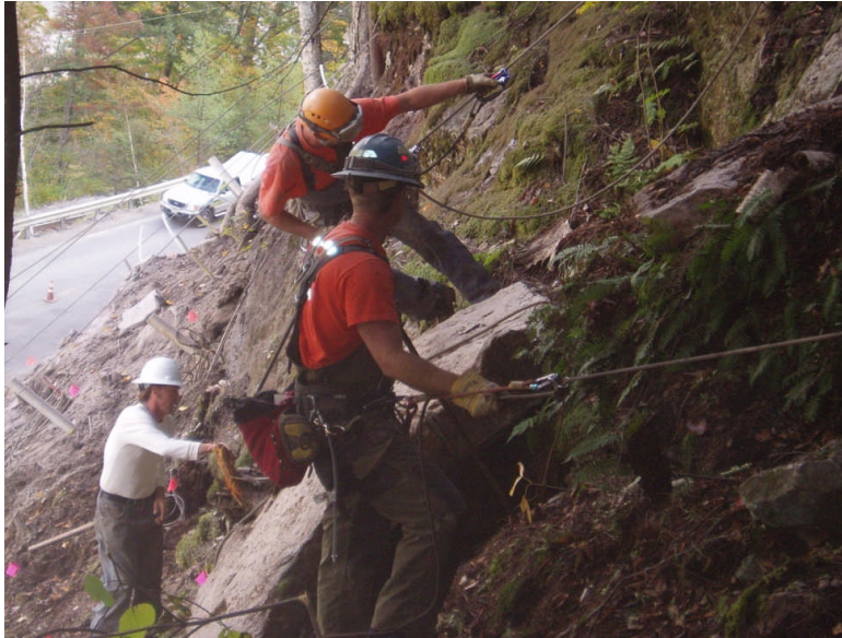
Figure 9. Workers tied off on the slope, clearing trees and scaling loose rock to prepare the slope for excavation and soil nail installation. Photo by K. Breskin.
