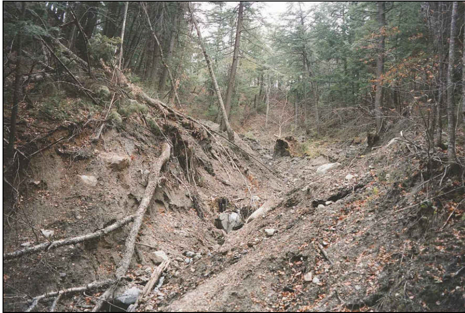
Figure 12. Scar from landslide of July, 1998, in till along ravine on west side of Wild River valley. Photo taken November 3, 1998. From MGS Open-File Map 03-57 by W. Thompson.
