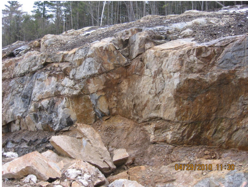
Figure 11. This rock cut slope at Stop 4-B experienced several rockfall events during the winter of 2010, after rock excavation shown on the plans was completed but before final remediation with drains and dowels. Photo by K. Breskin.
