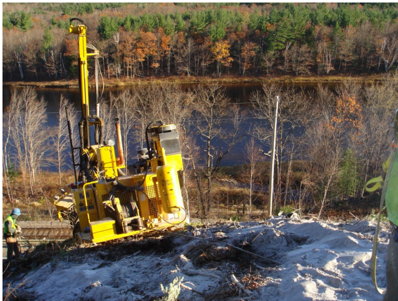
Figure 10. Rock cut slopes are high in this area, and rock was line drilled and pre-split to ensure long term stability of the slopes. Photo by K. Breskin.
