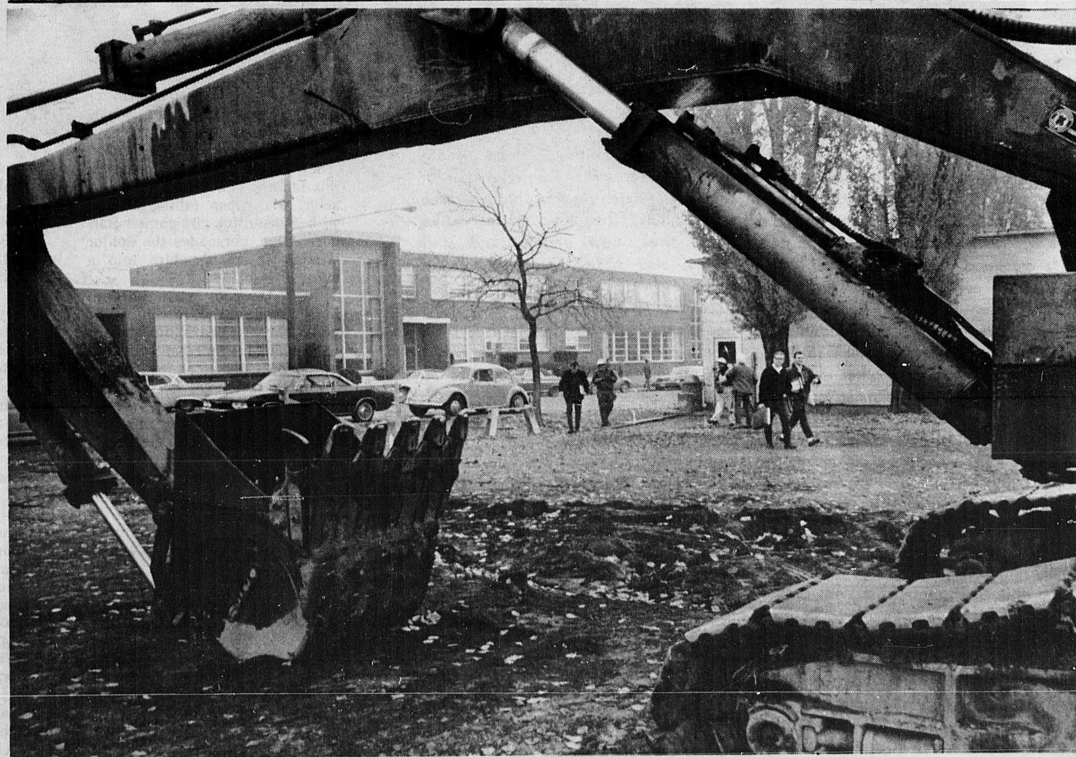
CONSTRUCTION ON PATTERSON HALL finally got underway last week in the area between the Music building and Twanka Commons. The scene above shows students using the short-cut across the mall for the last time as the construction crew fenced the area off shortly after beginning. (Photo by Joe Oakley).
