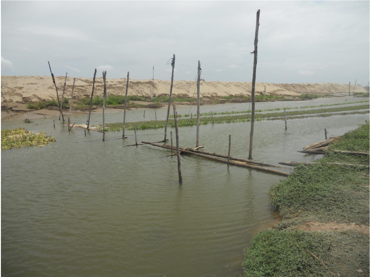
Figure 15. Sand filling in the wetland near site W8 for a development project.
