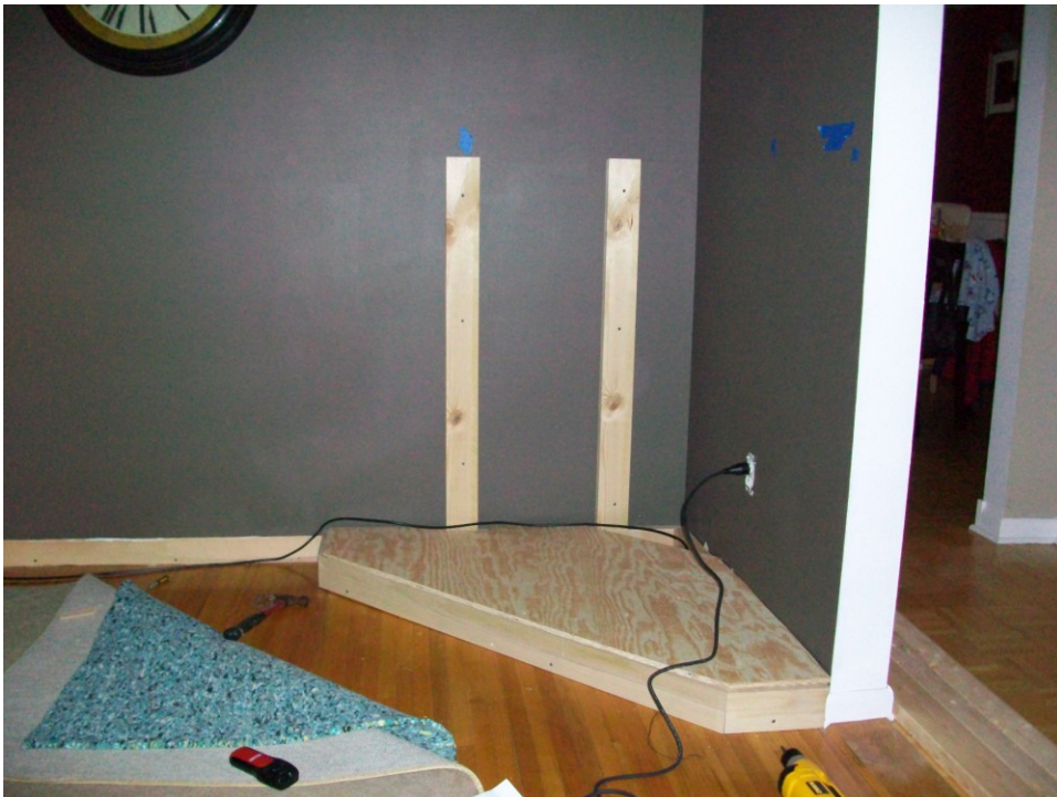
Figure B 4. The platform for the hearth is made of 1" plywood and 2x4 support beams were attached to studs in the wall.
