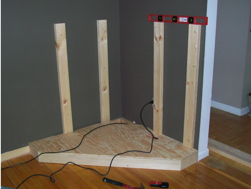
Figure B 5. Two additional support beams were attached to the studs within the walls. I checked to see that everything remained level.
