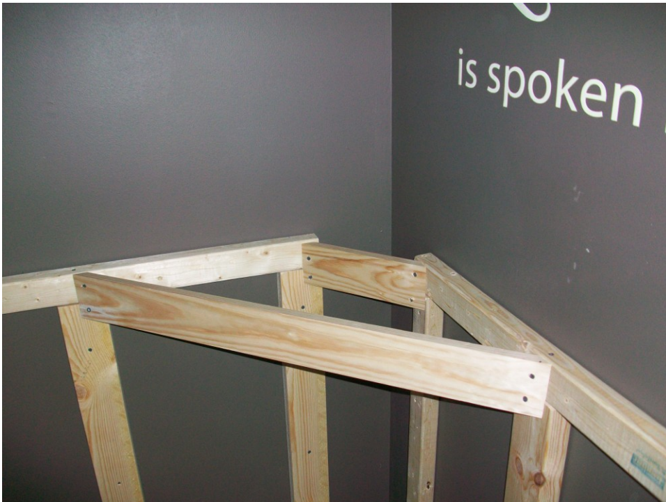
Figure B 10. Two diagonal support beams were added to reinforce plywood top. I did this so that the structure could withstand the weight of a television.
