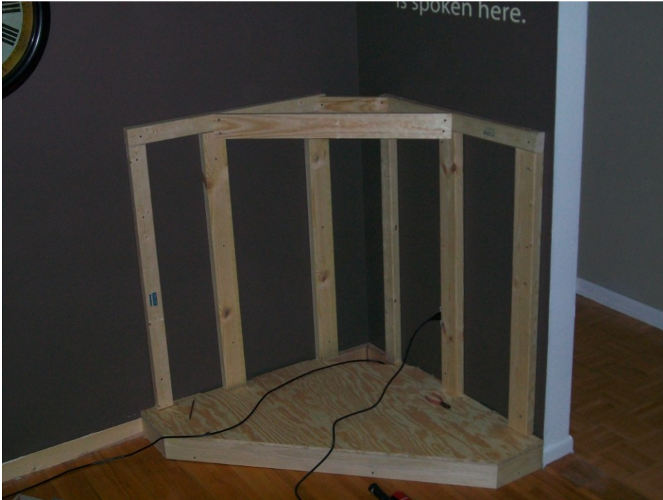
Figure B 11. This is the complete skeleton of structure. The outer panels are ready to be attached.
