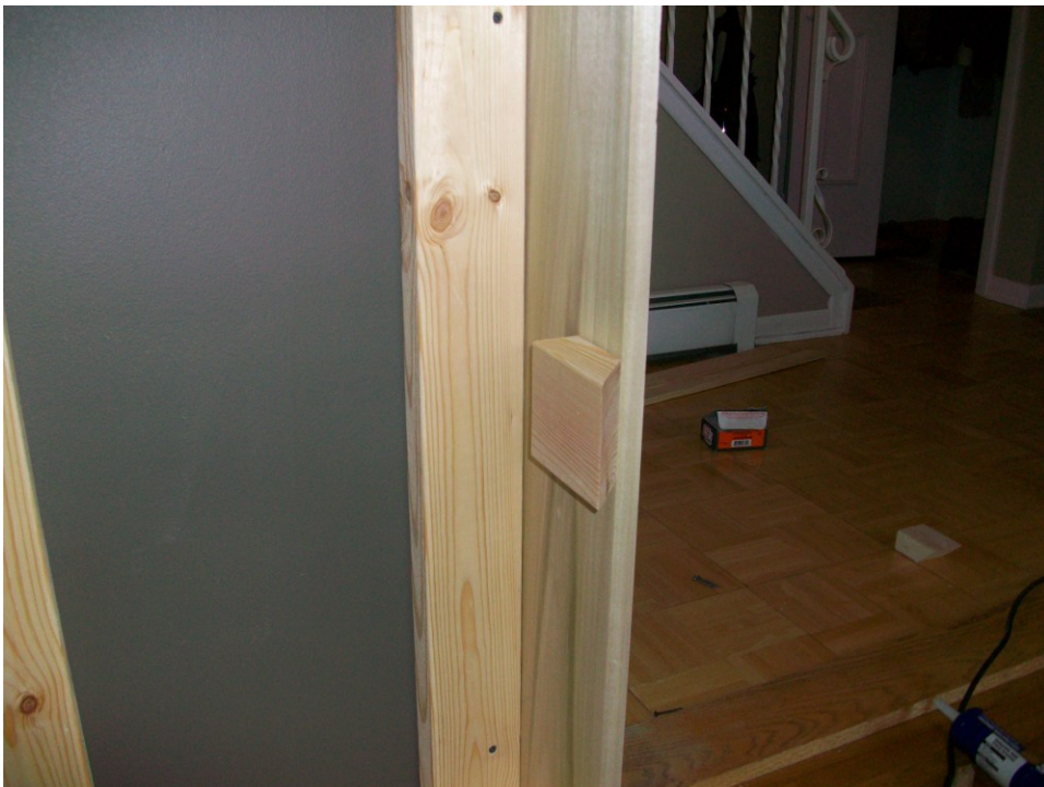
Figure B 16. When these brackets were screwed into the side panels, their 45 degree angle provided a flat surface to attach the front panel.
