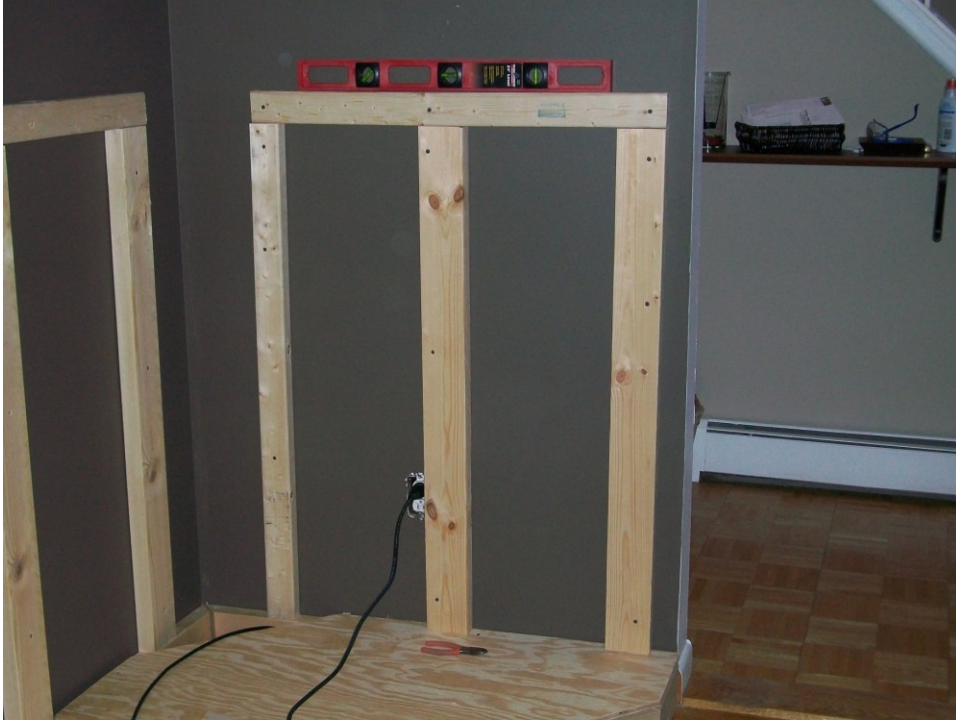
Figure B 9. I added horizontal beams to support the mantle's back edges.
