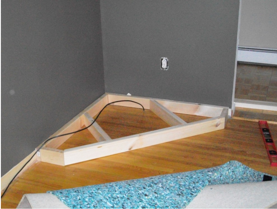
Figure B 3. This is the framework for the hearth, constructed from 2x4s.
