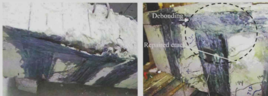
Figure 2.6: Typical CFRP debonding failure modes for the tested beams (Hussein et al. 2013)
