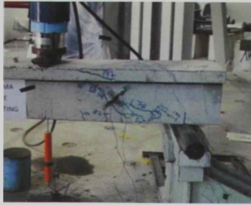
At peak load ( first shear test)
