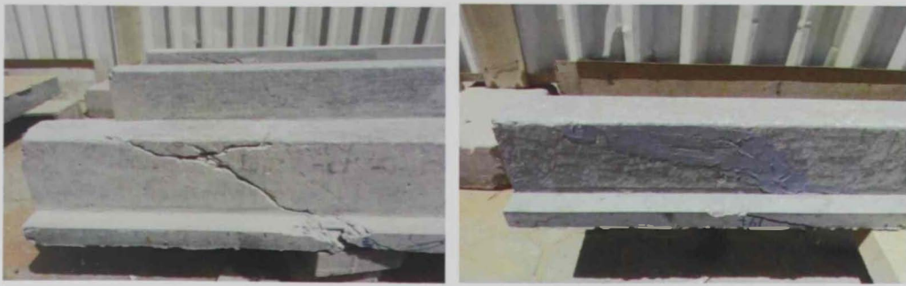
(a) Chasing-out of pre-existing cracks (b) After sealing of cracks and finishing of concrete surface
