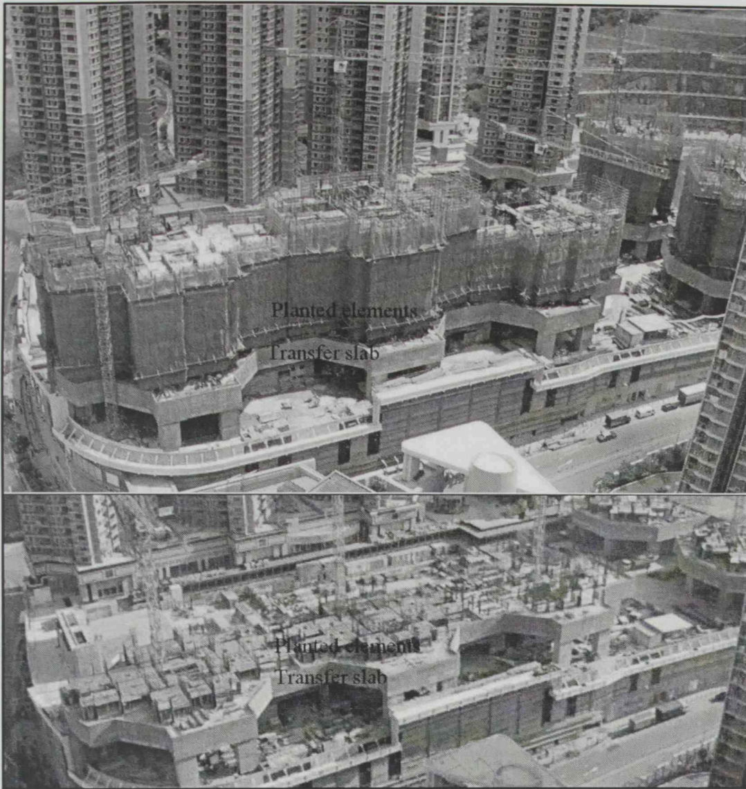
Figure A.10: Residential development in Tiu Keng Leng, Metro Town - building 11 (Wong, 2013)
