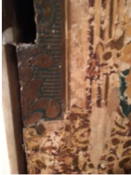
Fig. 25 Wallpaper fragment discovered during a renovation, likely French, 19th century, wood-block print. Home of Anne MacNeil, Elms Court, Natchez, Mississippi. Image courtesy of Anne MacNeil.
