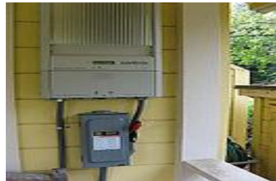
Fig. 3: A PV Inverter Installed in a Porch.
