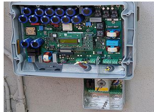
Fig. 1: Internal View of a Solar Inverter.
