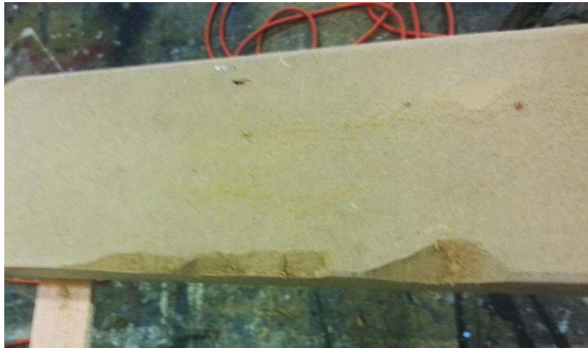
Figure 33: Schultz Window Distressing
