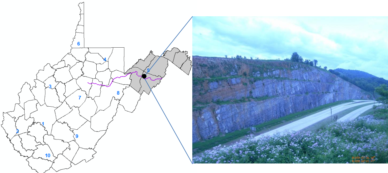
Figure 6.1 Slope Section of US Rt. 48 (Corridor H) in WVDOT District 5, Grant Co., WV
