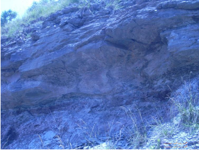
Photo 1: Large undercut from Redbed shale erosion below more competent rock strata at Location 4.
