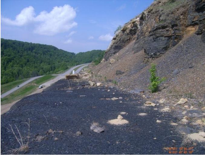
Photo 1: Large amounts of siltstone erosion on benches at Location 3.
