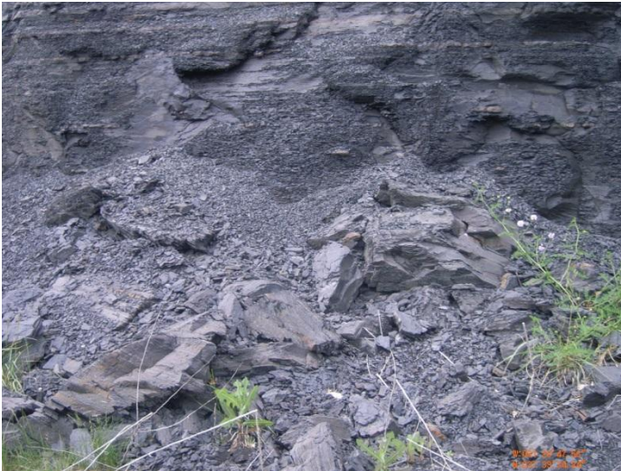
Photo 2: Larger fallen rocks from localized failure on upper bench at Location 3.
