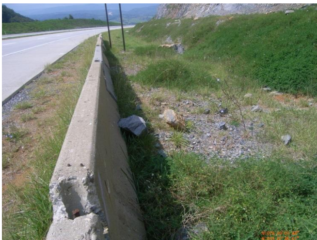
Photo 3: Jersey barrier and small catchment ditch at toe of slope at Location 1.
