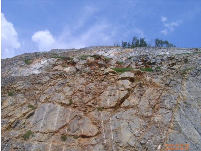
Photo 1: Fractured backslope face with clay infilling at Location 1.
