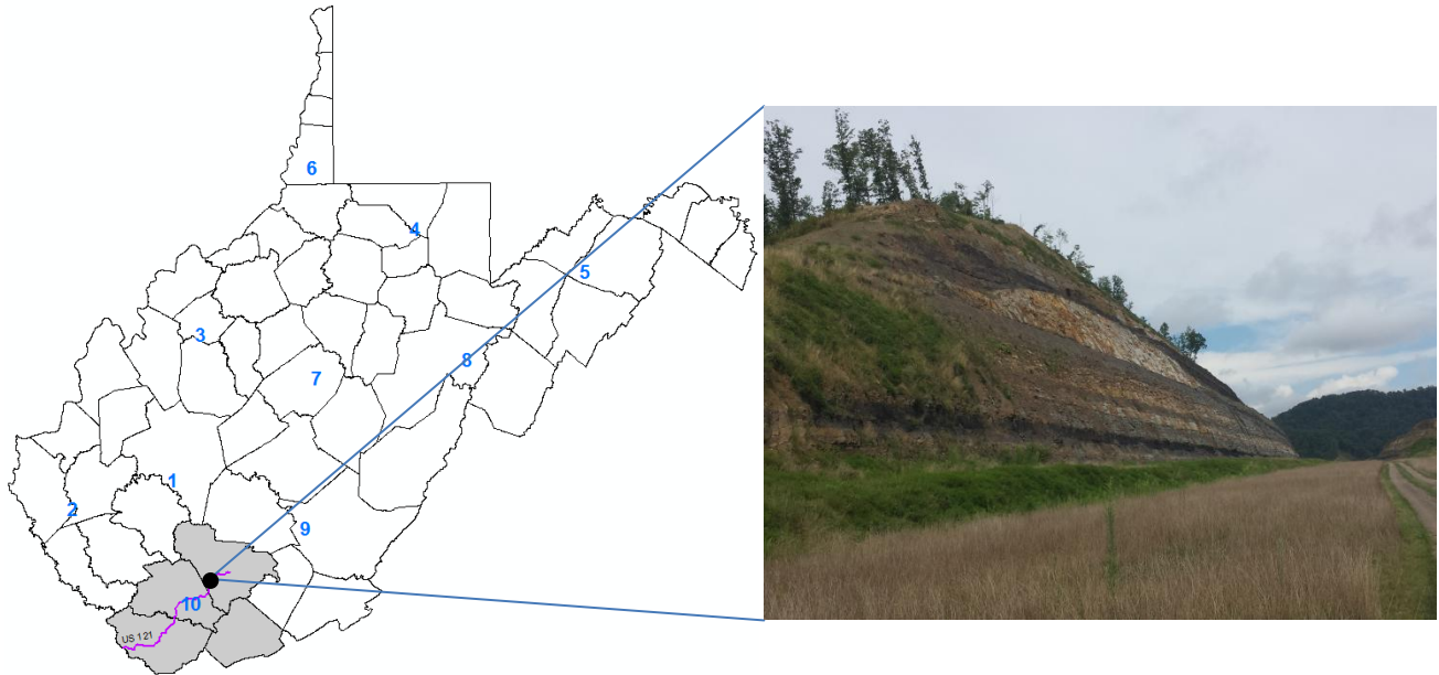
Figure 6.3 Slope Section of US Route 121 (Coalfields Expressway) in WVDOT District 10, Raleigh Co., WV.
