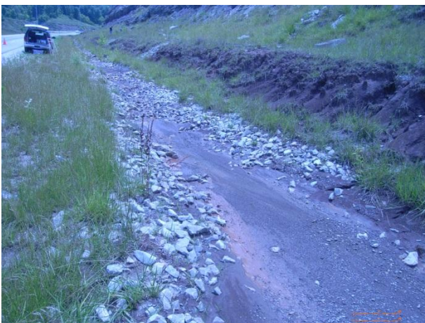
Photo 3: Drainage ditch at toe of slope, filling with eroded material at Location 4.
