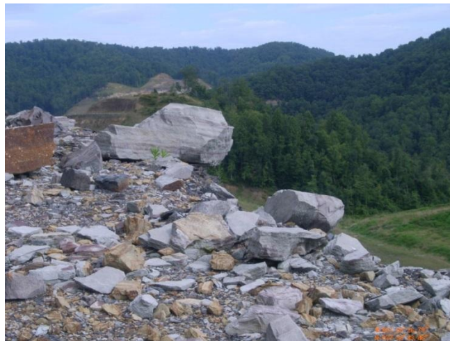
Figure 6.4 Accumulation of large rocks on a bench on the US Rt. 121 Cut Slope Section
