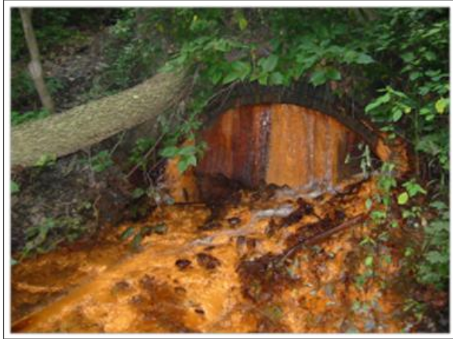
Figure 1.1 — Mine discharge portal at Iron Falls in Allegheny County, PA. The portal was sealed in the late 1960s and since then has been discharging alkaline mine drainage into the Youghiogheny river.
