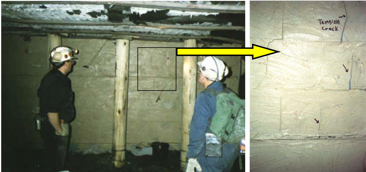
Figure 6-15. Damage of a stopping caused by roof-to-floor convergence of a mine entry.
