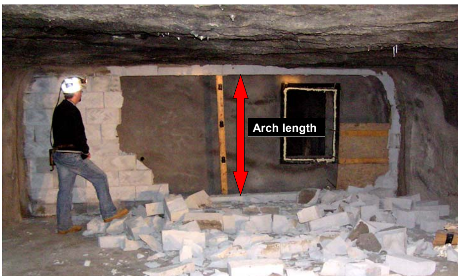
Figure 4-15. Arch height shown to occur between top and bottom layer of block that were grouted (cemented) in place in this particular test.
