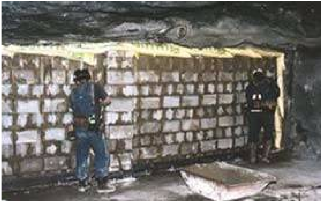
Figure 6-29. Installation of seal with preloading grout bags used to seal around the perimeter of the block wall.
