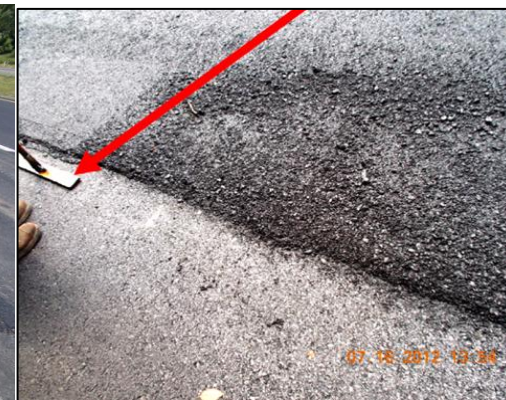
Poor - Pushing material too far at longitudinal joint (Project Id 74)
