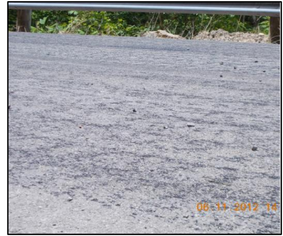
Poor (Project Id 122)
