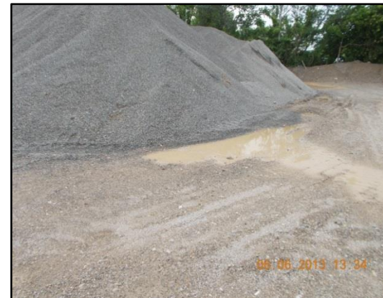
Poor base condition (Project 158)
