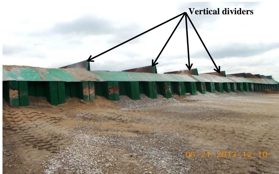
Figure 2-8 Vertical dividers (Dunbar asphalt plant in WV)
