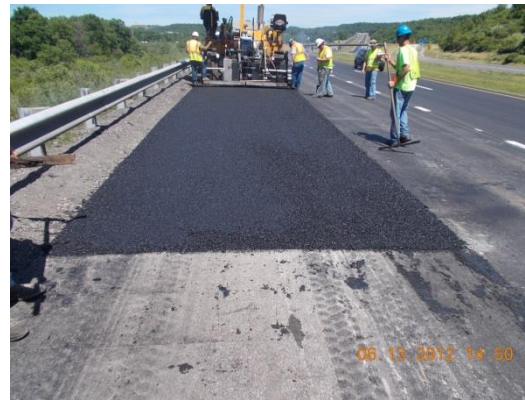
Fair - Luting should be minimized for transverse joint (Project Id 57)
