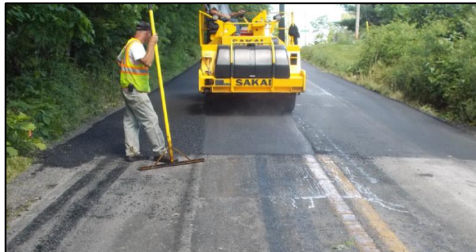
Poor Compaction parallel to paving direction (Project Id 38)
