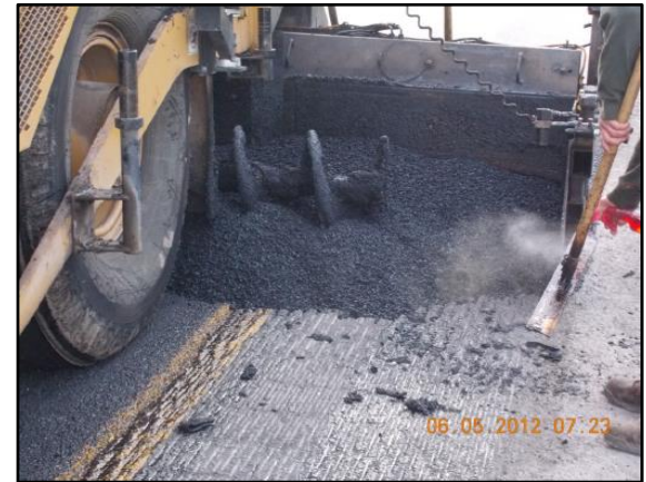
Poor (Project Id 52)
