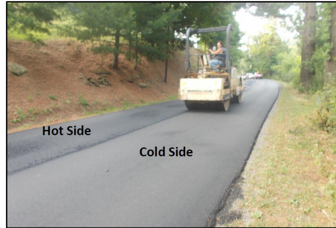
Poor roller placement cold-to-hot (Project Id 93)
