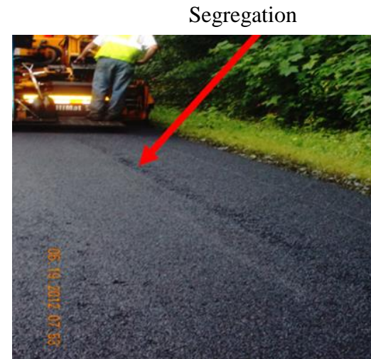
Poor (Project Id 122)
