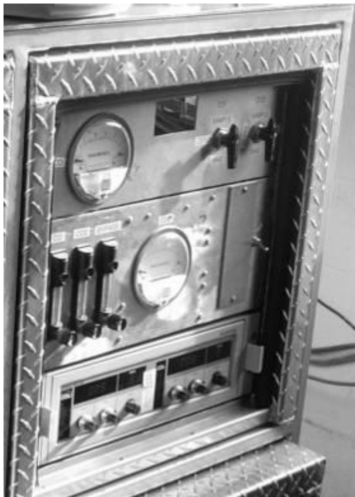
Figure 30 - CO/CO 2 Analyzer and Flow Control
