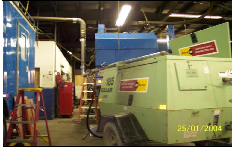
Figure 6 SullAir 185 Diesel Powered Air Compressor
