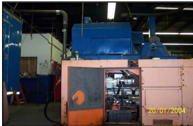
Figure 5 Side View of the Multiquip-Whisperwatt Generator
