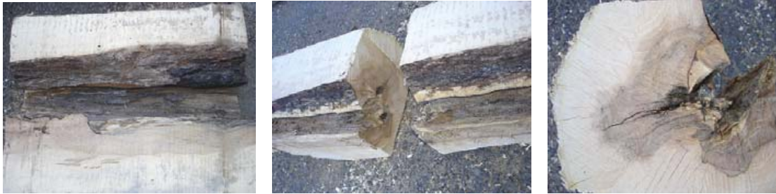
Figure 1-2 Decay or rot in wood (Agrawal 2005)
