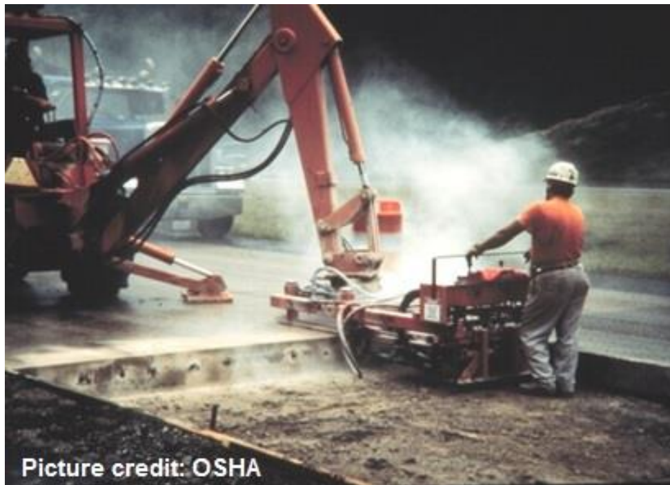
Figure 46: NOA or Asbestos?
