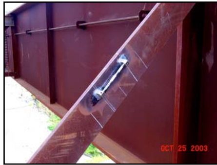
Figure 4.11 Strain Gage Bonded to a Diaphragm Diagonal Member
