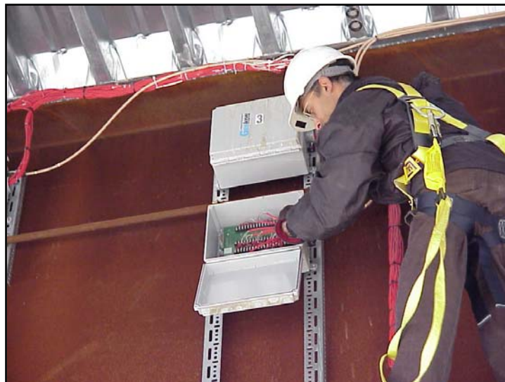
Figure 4.20 Wiring of Gages to Multiplexers Boards
