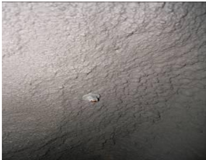
Figure 5-4. Post Blast Picture of a leaky feeder cable hung perpendicular to entry in Lake Lynn Laboratory (“I-bolt” sheared off from explosion, Leaky Feeder destroyed)
