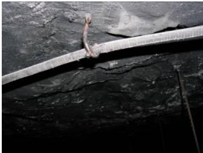
Figure 5-2. Post Blast Picture of a leaky feeder cable hung parallel to entry in Lake Lynn Laboratory (“J” hook melted to cable)
