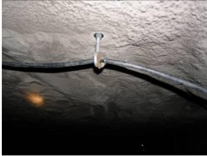
Figure 5-3. Pre-Blast Picture of a leaky feeder cable hung perpendicular to entry in Lake Lynn Laboratory
