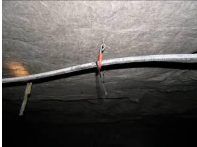
Figure 5-1. Pre-Blast Picture of a leaky feeder cable hung parallel to entry in Lake Lynn Laboratory
