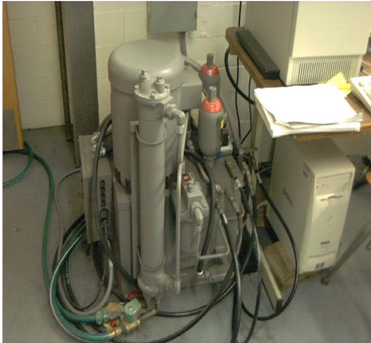
Figure 4.2 Hydraulic Power Supply
