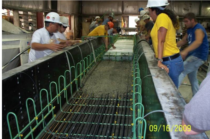
Figure 4-3 Picture of concrete, void and upper rebar placement during traditional beam casting.
