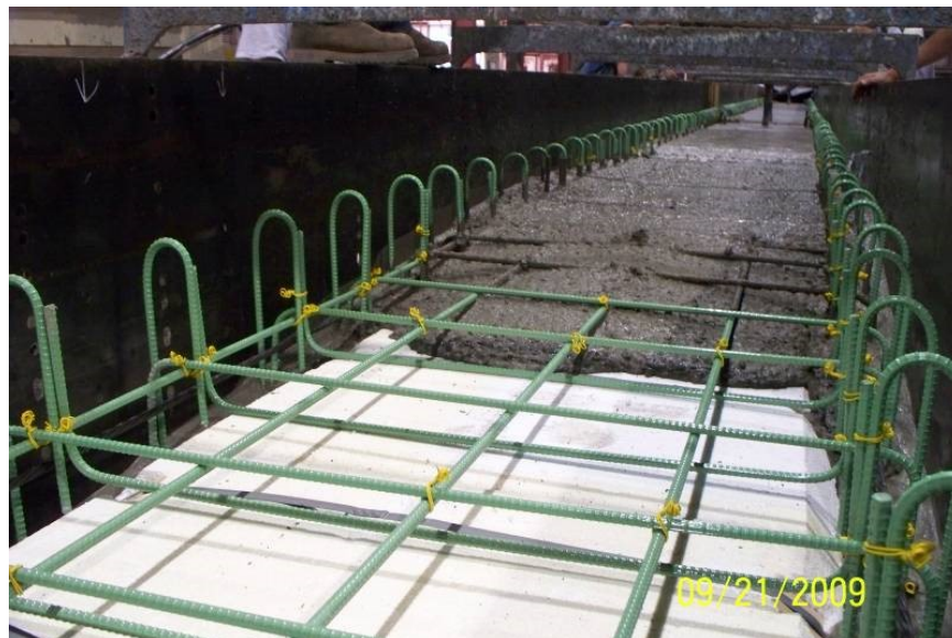
Figure 4-4 Pre-assembled formwork during placement of concrete in single lift for SCC-2 beams.
