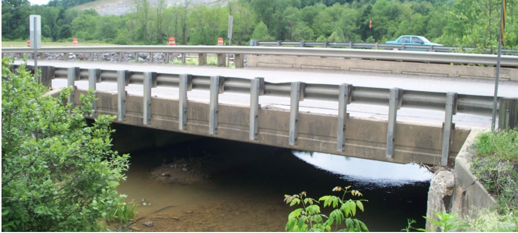
Figure 1-1 Old Stalnaker Run Bridge, with temporary bridge in background. View from upstream location.
