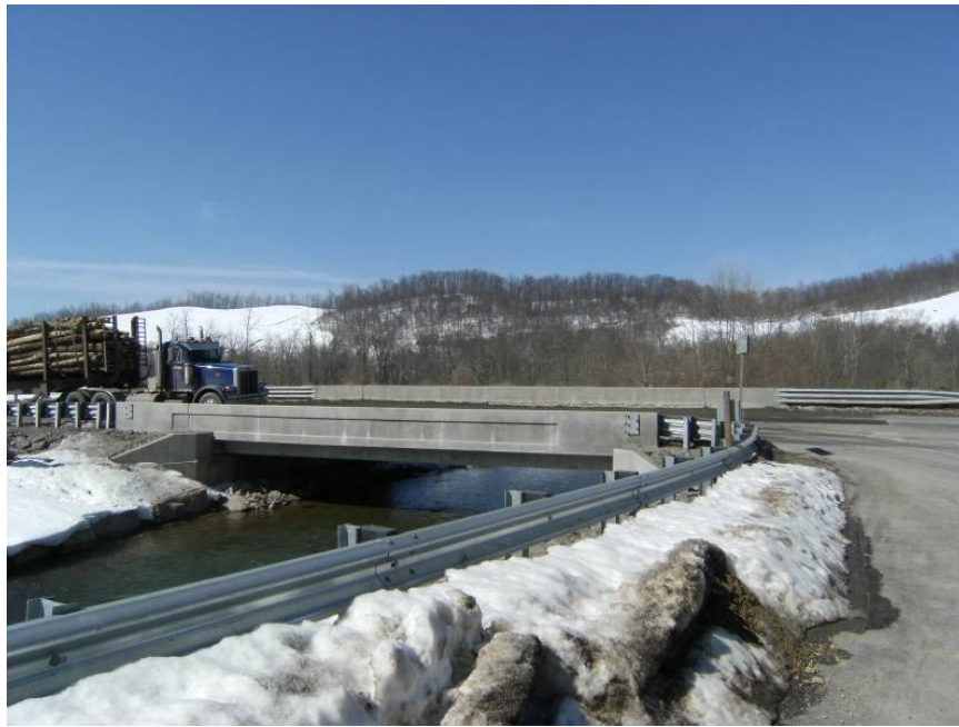
Figure 5-3 Stalnaker Run Bridge replacement after completion; View from Stalnaker Run Road (upstream, north bank).
