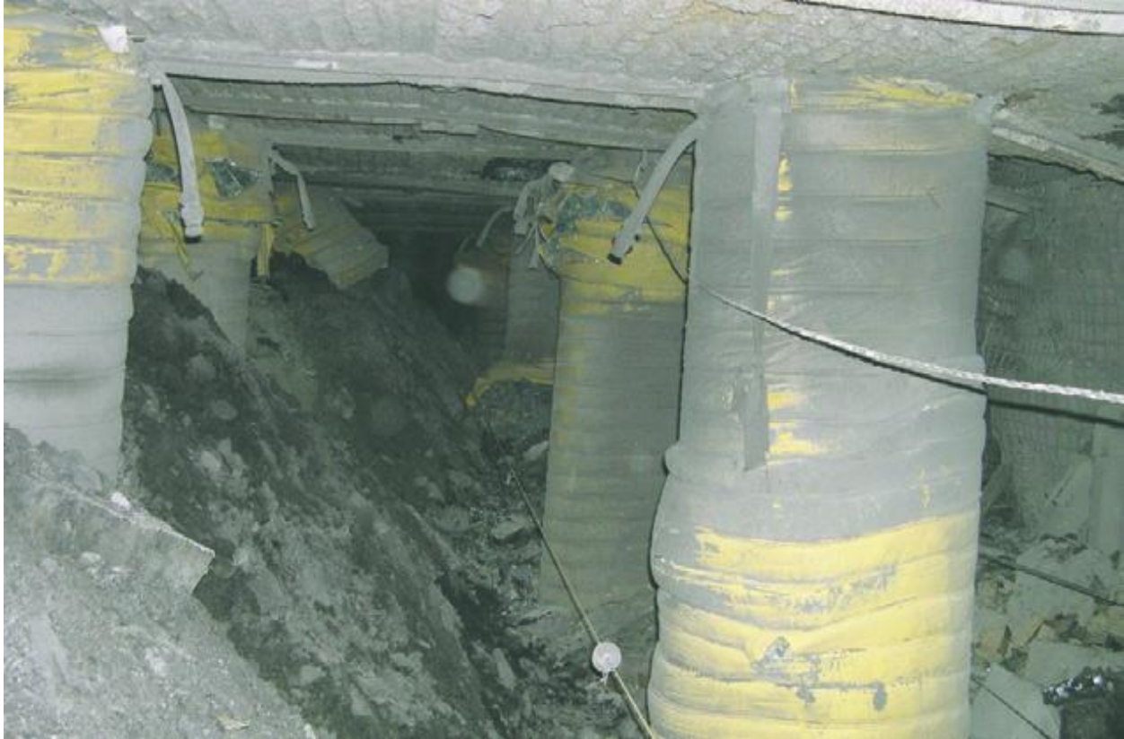
Figure 2-26. Pumpable cribs in tailgate entry inby the longwall face, looking inby showing a low resistance ventilation pathway into the gob (Zhang, 2012).
