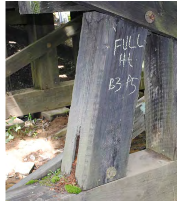
Bent 3 - Post 5 Rot
