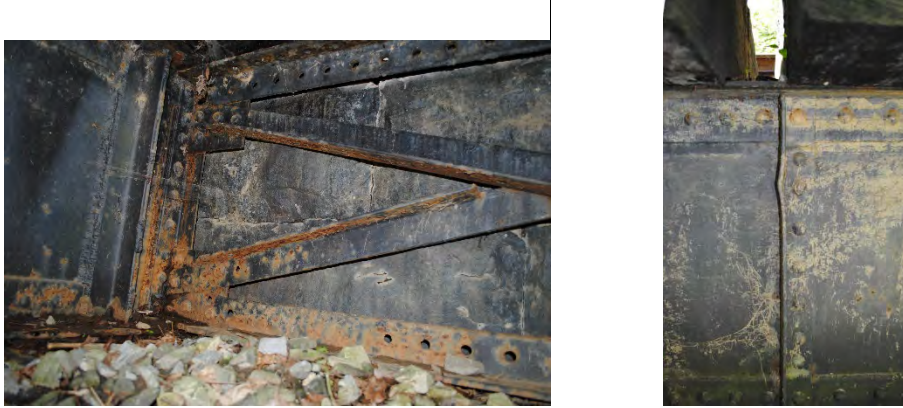
Figure 52 - Bracing corrosion (left) and bend in web stiffener (right)
