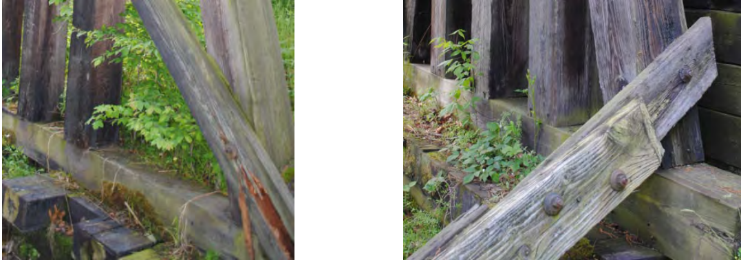
Figure 39 - Bent 6 Sway Brace split/rot (left) and West Tower Brace 4 splice (right)
