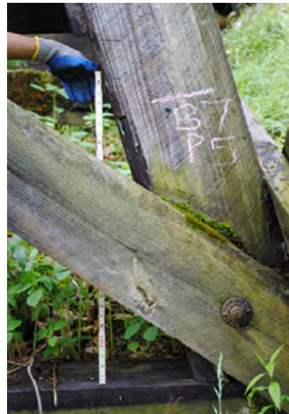
Bent 7 - Post 5 Rot
