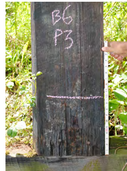
Bent 6 - Post 3 Rot
