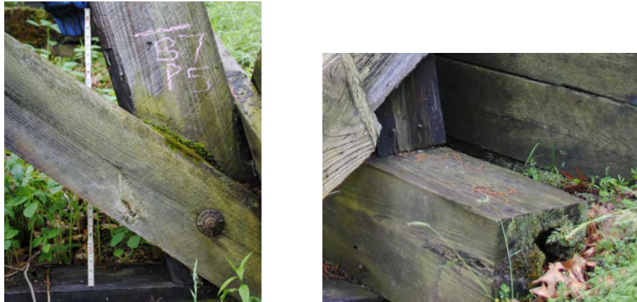
Figure 37 – Bent 7 Post 5 (left) and Bent 8 Sill end rot (right)
