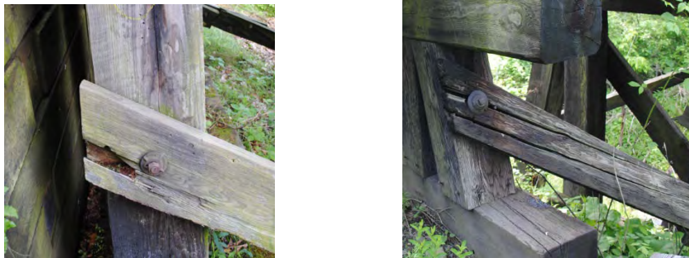
Figure 38 - East Tower Brace 4 rot/split (left) and West Tower Brace 1 split (right)
