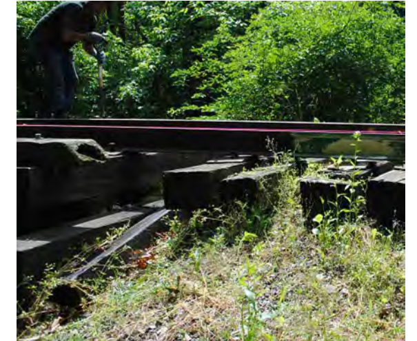
North Approach Poor Condition
