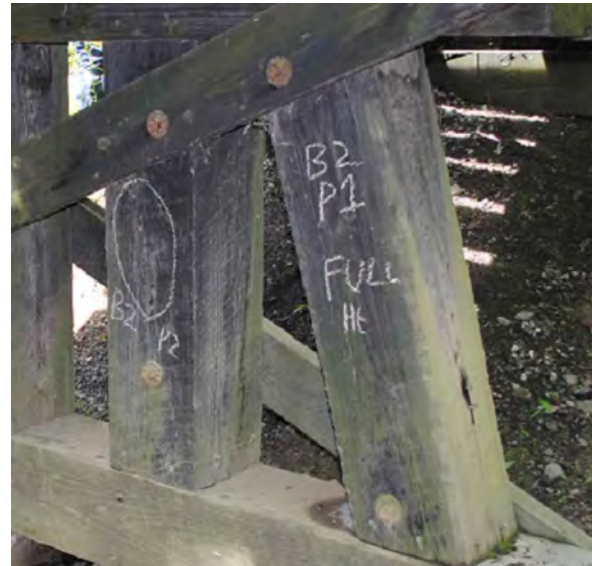
Bent 2 - Posts 1 & 2 Rot
