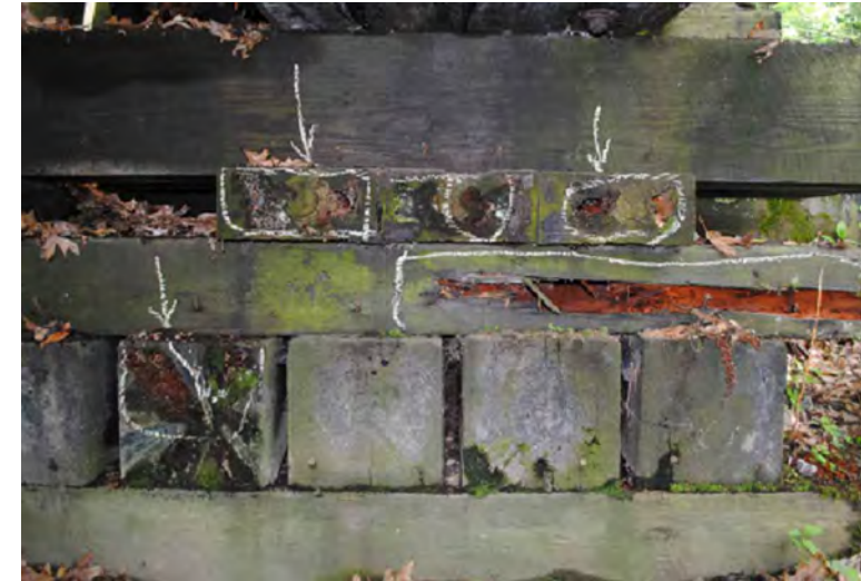
Bent 4 - Rot in Blocks and Sill
