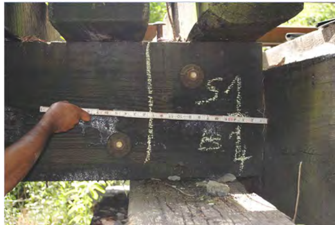
Span 1 - Stringer 1 Rot
