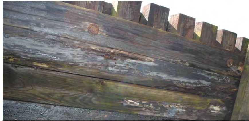
Span 3 - Stringer 2 Rot
