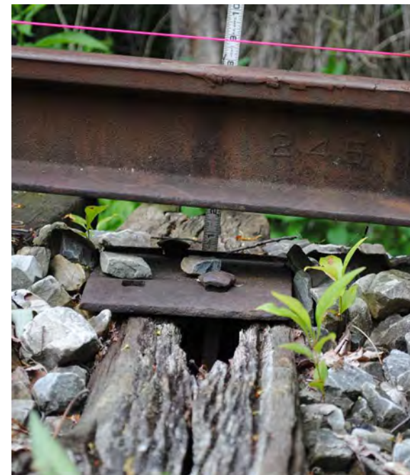
North Approach Low Ballast and Rot Tie
