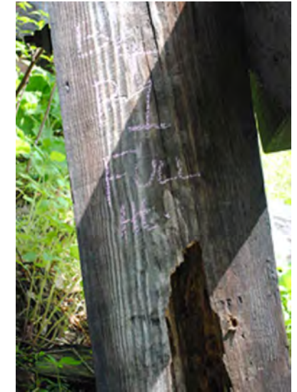
Bent 4 - Post 1 Rot
