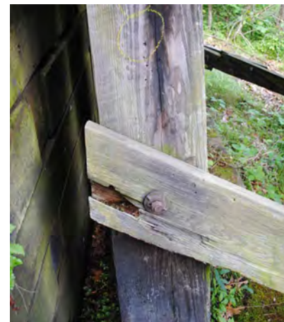
East Tower Brace 4 - Rot/Split
