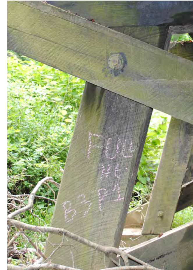
Bent 3 - Post 1 Rot
