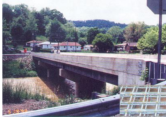
Figure 7.2 McKinleyville Bridge with Concrete Deck Reinforced with FRP Rebars, Brooke County, WV, Built in 1996
