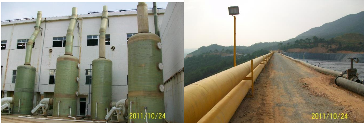
Figure 7.12 Extensive Uses of FRP Vessels and Pipelines at Zijin Mining Group, Shanghang, Fujian, China
