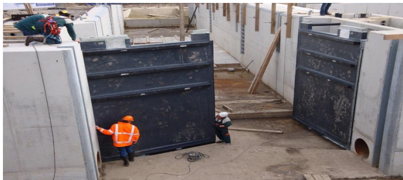
Figure 8.12 Eric Ter Apel Lock Doors
