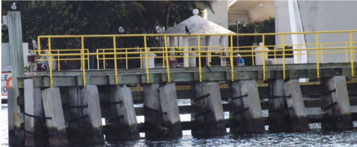
Figure 8.33 Strongwell's round SAFRAIL™ industrial handrail system in Fort Lauderdale, Florida
