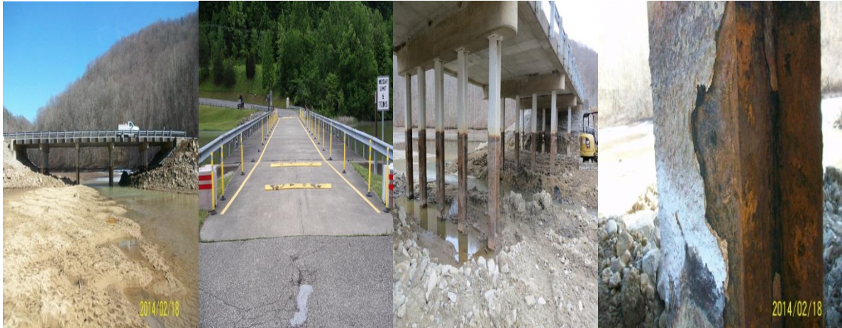
Figure 8.9 East Lynn Bridge Rusted and Scoured at Mudline
