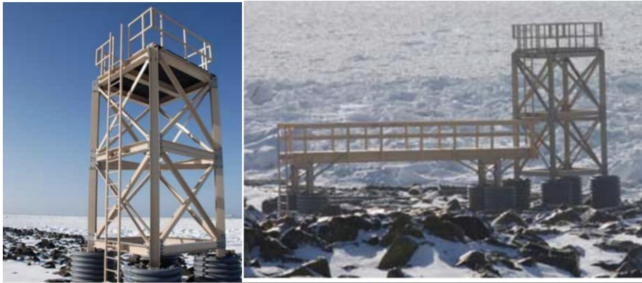
Figure 8.24 FRP arctic towers for a Seal Observation Facilities Project on St. Paul Island, Alaska
