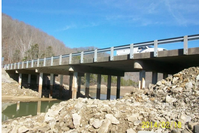
Figure 9.13 East Lynn Lake Bridge with severely corroded steel structural members, Cove Creek, West Virginia
