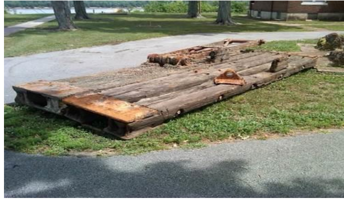
Figure 8.5 Deteriorated Wood Wicket Gate Pulled from Service
