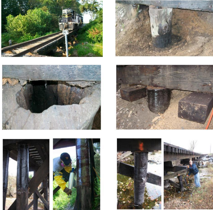
Figure 7.19 Retrofitting of Railroad Bridges Using FRP Wraps without Interrupting Railroad Service, SBVR, Moorefield, WV (July 2010)
