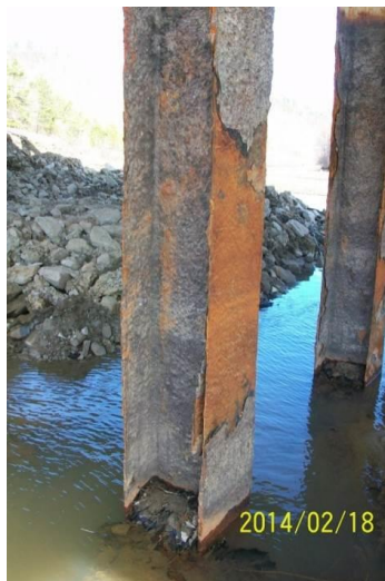
Figure 9.14 Close-up of corroded steel pile
