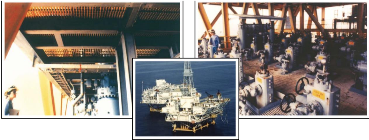
Figure 8.20 All-fiberglass well bay deck for 18 wellheads on Shell's Southpass 62A production platform
