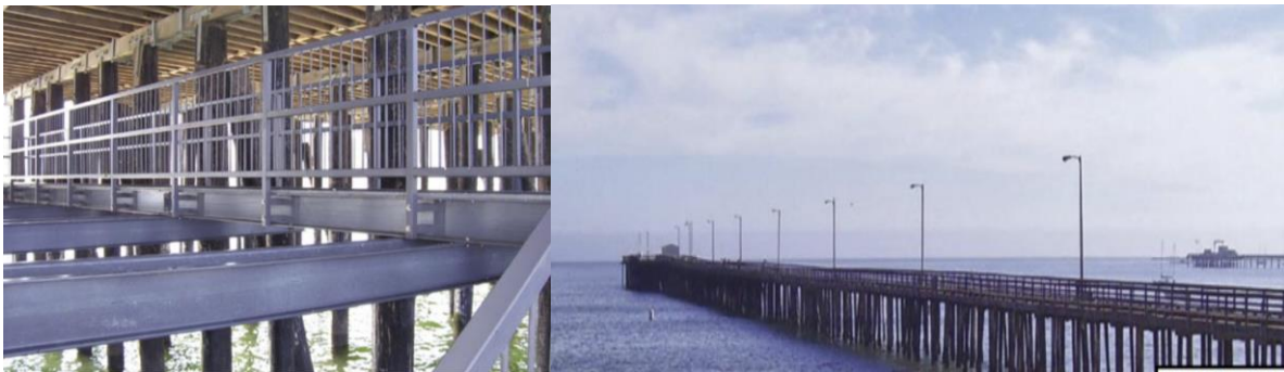
Figure 8.23 The Avila Beach Pier in California reconstructed using Strongwell's pultruded fiberglass structural materials
