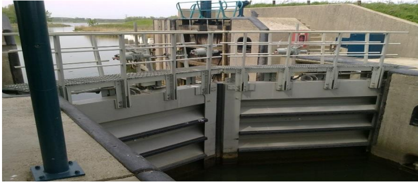
Figure 8.11 Werkendam FRP Lock Doors
