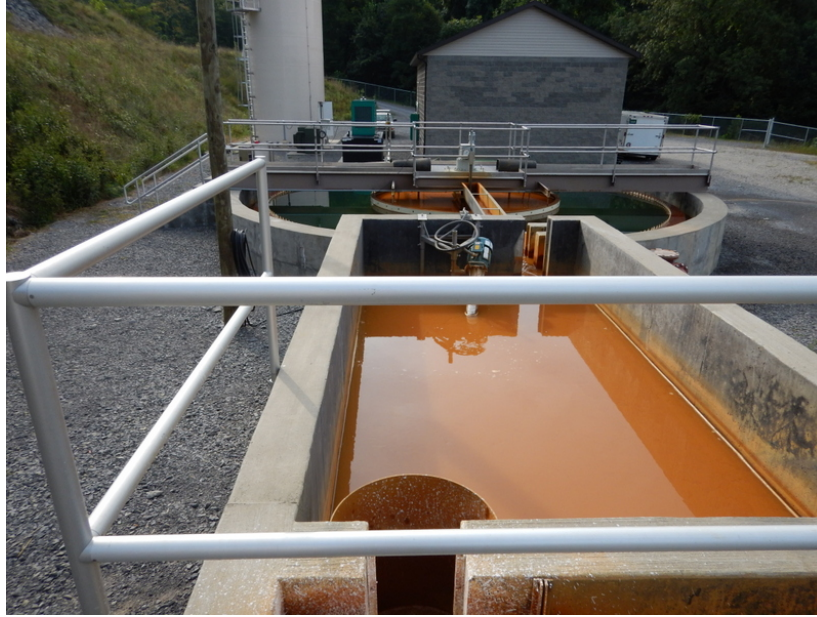
Figure 1.4 – Small clarifier used for treatment of AMD. The foreground shows the area where alkaline material and aeration is used to raise the pH. The clarifier structure is located in the middle while the lime storage silo is located in the background.
