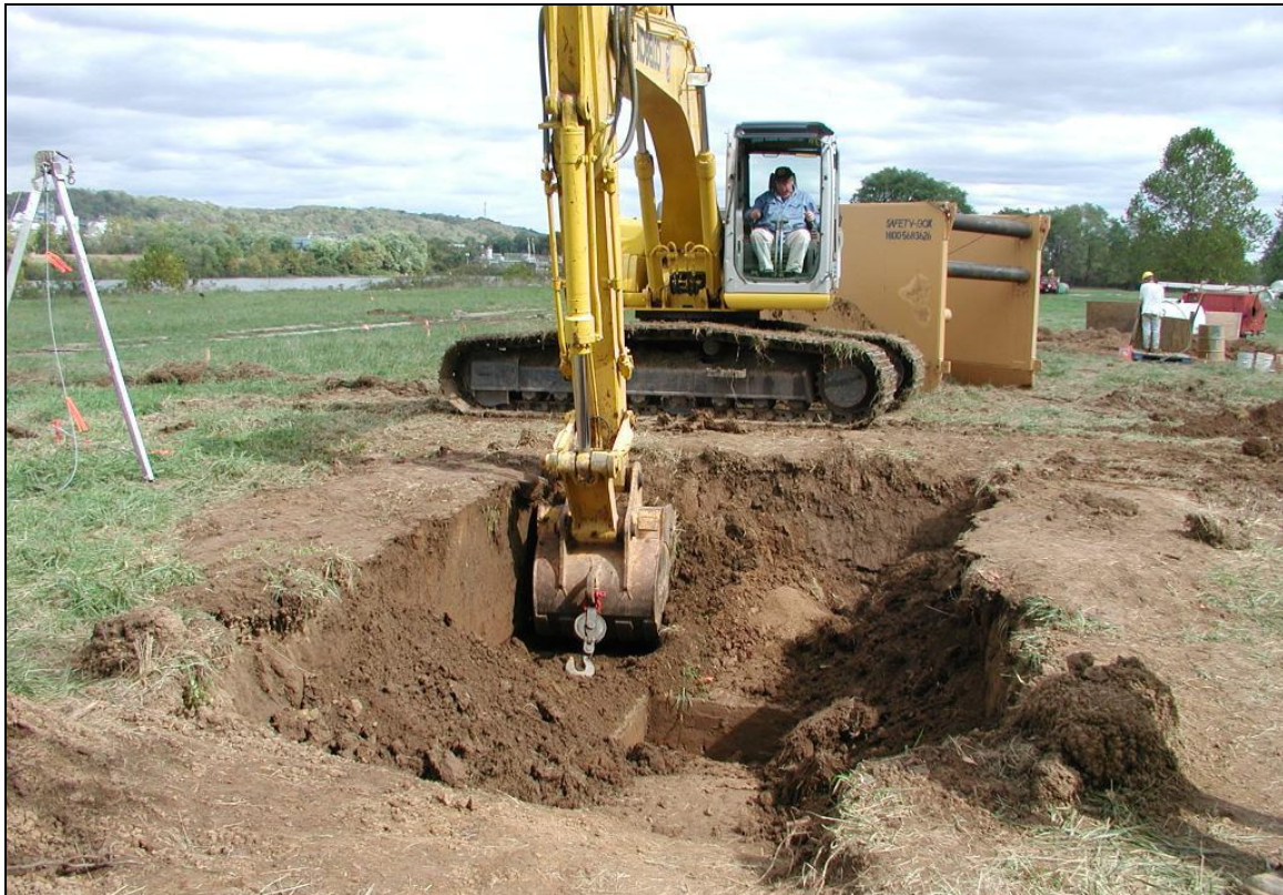
Figure 10: View of Deep Test 2 facing northeast on 5 October 2002. Note the 1 m x 1 m test unit N460 E500 at the center of the trench, the trench box behind the tracked excavator, and the north channel of the Ohio River, flowing downstream to the left, in the left background of the photo. From Robinson et al. 2008.
