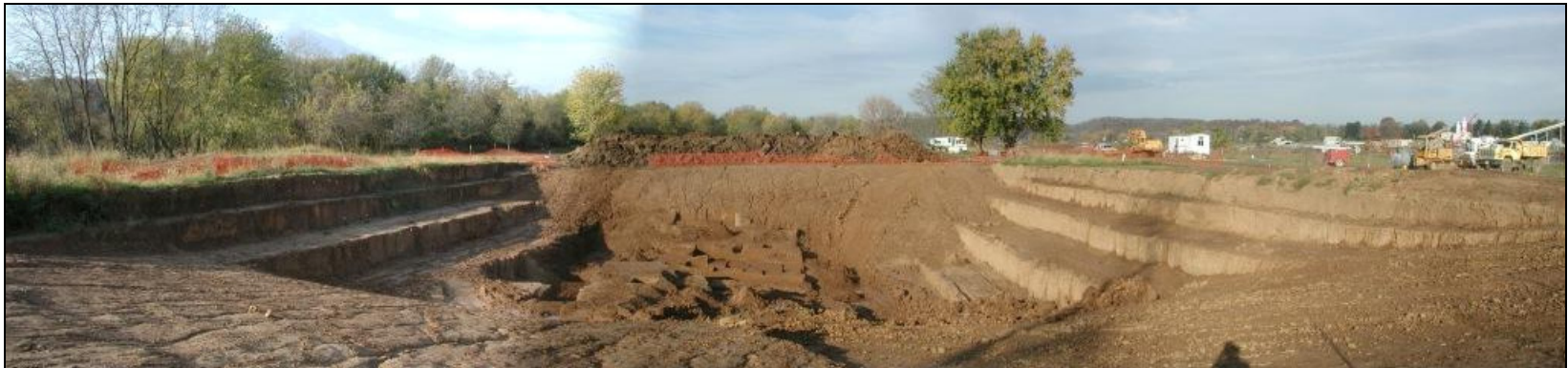
Figure 32: View of Pier 5 excavated to CS V, facing downriver (west) on 31 October 2003. Photo shows Pier 5 upon completion of excavations, immediately prior to backfilling.
