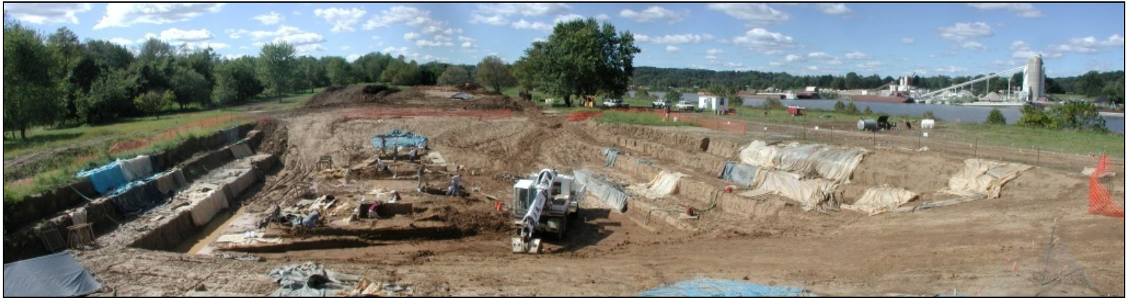
Figure 31: View of Pier 5 excavated mid-way through CS IV, at the levels of OC 2 and OC 2A, facing slightly right of downriver (west-northwest) on 2 October 2003.
