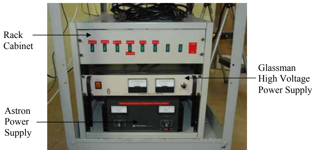
Figure 3.37: Glassman High Voltage Power Supply Addition Mounted in Cabinet with Astron Power Supply
