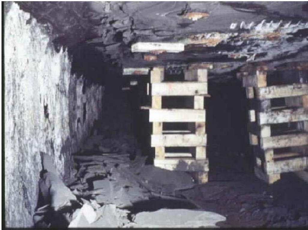
Figure 4.2. Cutter roof failure along one rib side of an entry [2].
