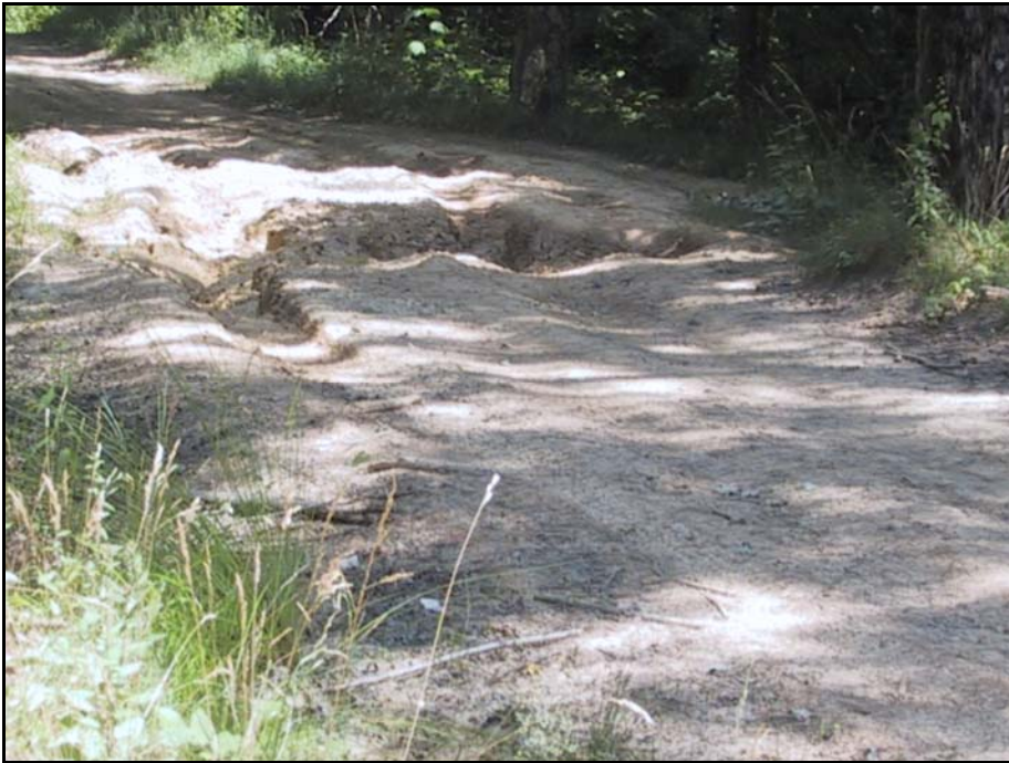
Figure A.3. Poor application of cross drainage in a haul road.
