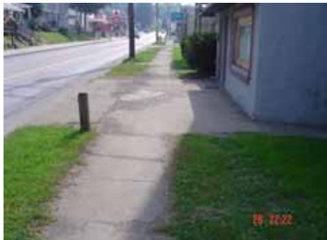
(c) Older-deteriorated surface
