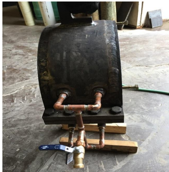
Figure 5-23: Inlet valves connected together.
